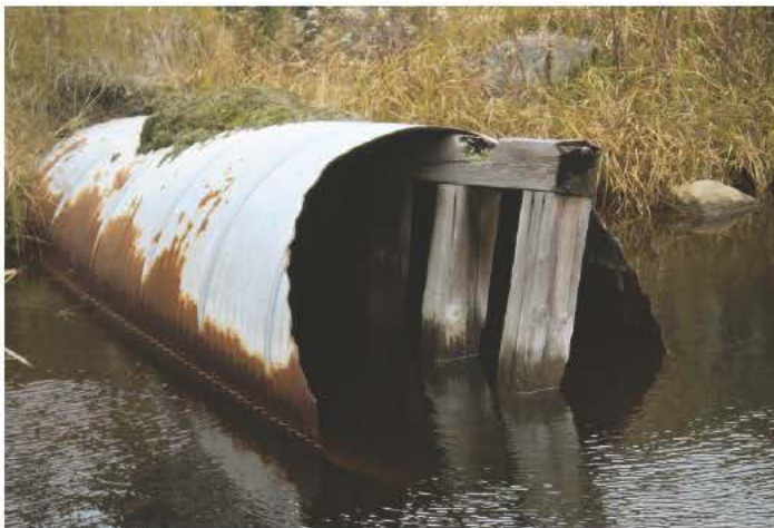
Deteriorated culverts under Trans Canada Highway
