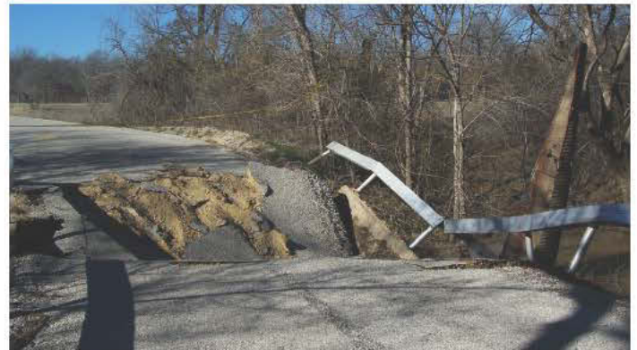
Crater caused by the corrugated steel pipe failure A section of the CSP is visible on the right hand side of the picture projecting vertically photo credit: John Dutschmann, Technical Resource Manager Hanson Pipe and Precast
