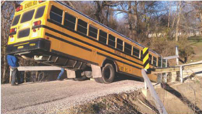
A school bus in a crater caused by a collapsed corrugated steel pipe photo credit: Dustin Hood
