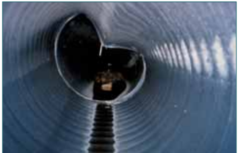
Failed Pipe Wall Buckling.
