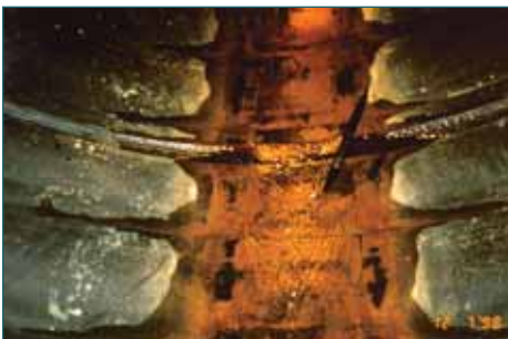
Cracked HDPE Liner.
