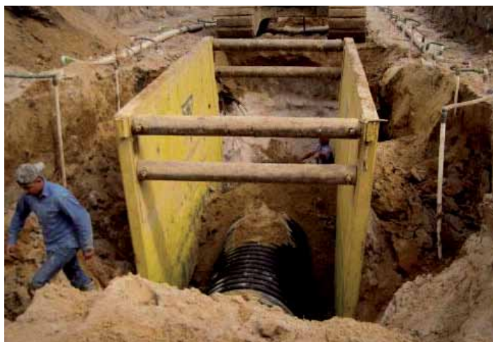
Safety versus proper installation 3.3 km of HDPE pipe ranging in size from 750mm to 1500mm failed on this project and had to be replaced
