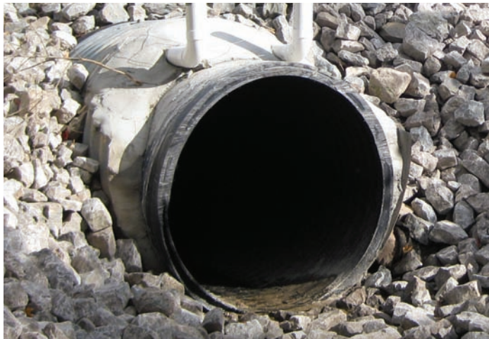
Relined culvert - reduced cross sectional area. This CSP culvert under Highway 407 in Ontario was relined after less than 20 years in service. The designer specified the appropriate rip rap protection to prevent erosion.
