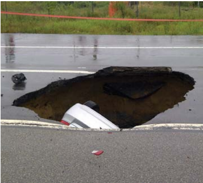
Car falls into Highway 174 sinkhole after steel culvert collapses underneath Courtesy: Ottawa Fire Services
