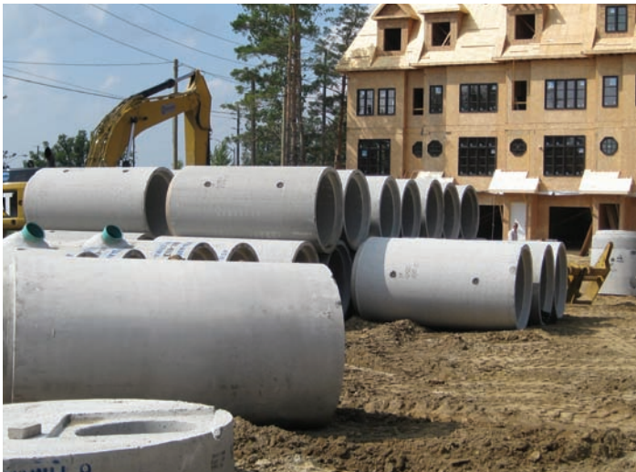
Ontario Building Code (OBC) requirements for a drainage system constructed in conjunction with a building are complex. It is critical that design professionals gain a firm understanding to specify code-compliant pipe products.
